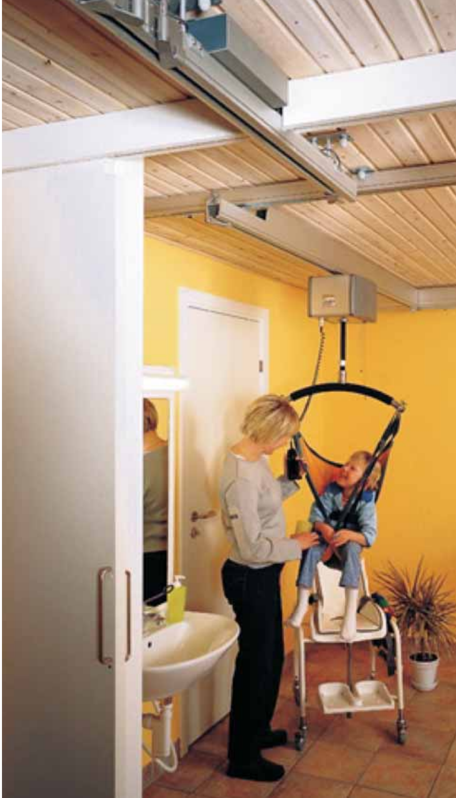
A ceiling-lift installation will help caregivers transfer family members with mobility impairments. The lift is motorized to move up and down and also forward and back. The tracks can be suspended from the ceilings or walls.
